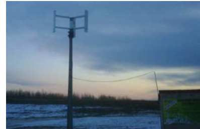
Figure 6. Micro-Wind Pilot Project in Grande Prairie, AB
